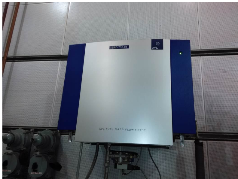
Fig 3.3 Fuel Conditioner System
