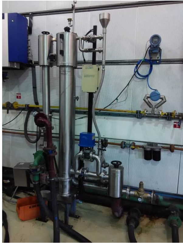
Fig 3.2 Coolant Conditioner System
