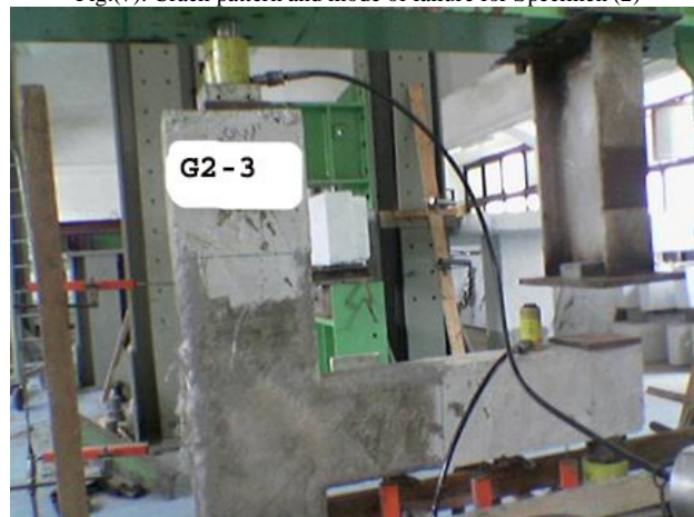
Fig.(8): Crack pattern and mode of failure for Specimen (3)
