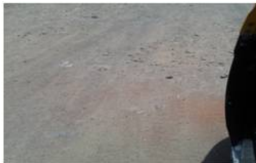
Fig.4 Bumpy road condition
