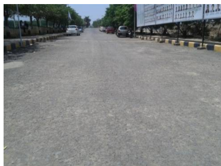
Fig.2 Rough road Condition
