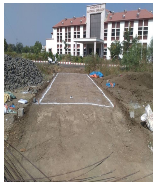
Fig.2 Constructed Artificial and Composite Subgrade of Model Flexible Pavement in Field for Present Study
