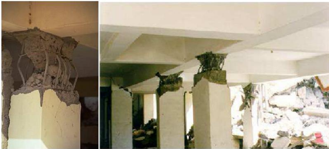
Figure.3 Damages in columns during earthquake
