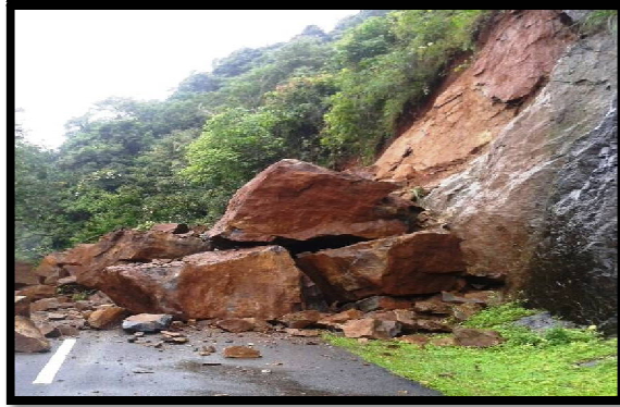
Fig. 5. Landslide along Madikeri-Virajpet road
