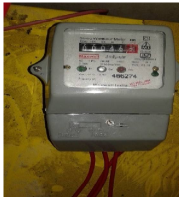
Figure (9): Energy Meter
