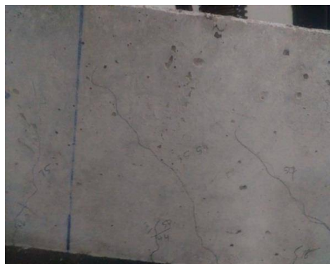
Fig 7.2 Crack pattern of 0.5% beam specimen
