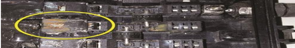
Figure 10(a): Corrosion in junction box
