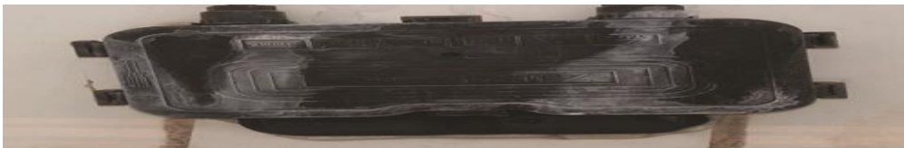
Figure 10(b): Moisture over the cover of junction box
