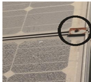
Figure 3(a): Corrosion on the interconnecting joints of solar modules
