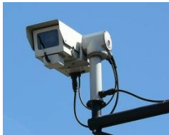
Fig.5: Wiper wipes the dust on camera
