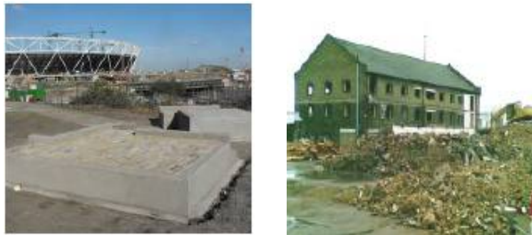
Figure 13: Reclaimed yellow stock bricks used to create seating areas on the Greenway and red and blue being reclaimed at Construction Zone B.
