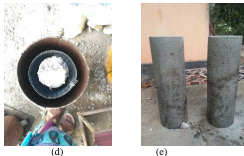
Fig.4. Procedure for jacketing column (a) Chipped column (b) Bonding agent(c)Chipped column coated with bonding agent(d)Mould ready for jacketing(e)Finished specimens
