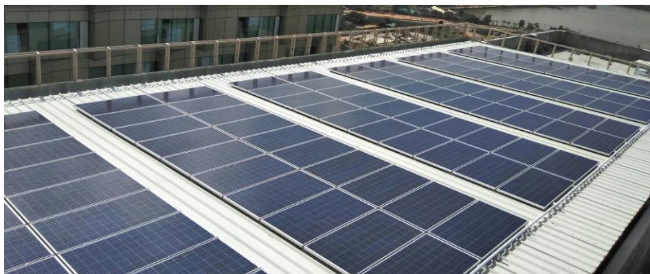
Fig-1: Solar PV plant installation on industrial sheeted roof top
