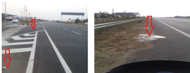
Figure 2. Road Accident Debris in National High Way
