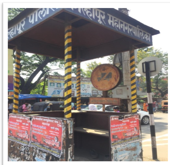
Fig 8 Poor maintenance of traffic signs
