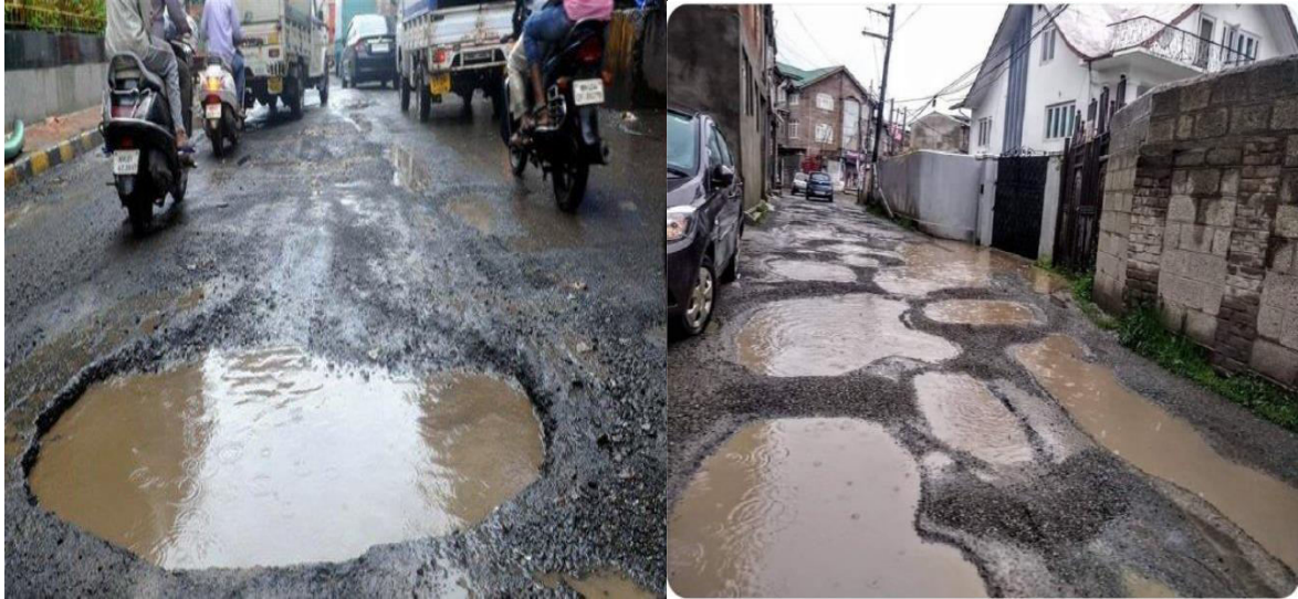
Dilapidated roads in the vicinity of Srinagar, Kashmir
