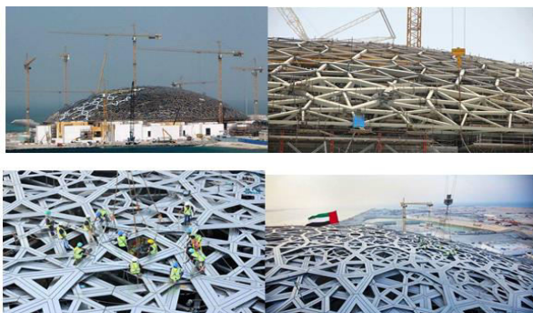
Fig.14 : The construction method used to raise the layers of the dome over buildings and streets
