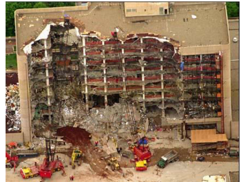
Figure 1(b)- Murrah Federal Office Building after 19 April 1995 attack.
