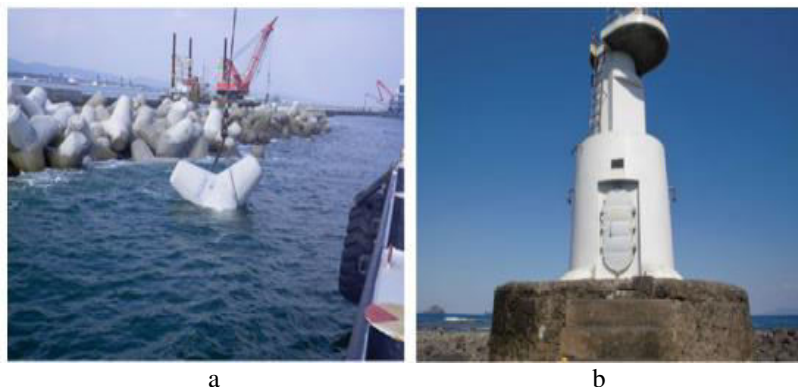
Figure 1: Shows a breakwater armour made from seawater mixing concrete (a) at Soma Port, Japan, and a lighthouse built in 1959 with reinforced Concrete made from seawater mixing Concrete (b) at Hizen Nagasaki Nao, Ukushima Island, Japan [58].
