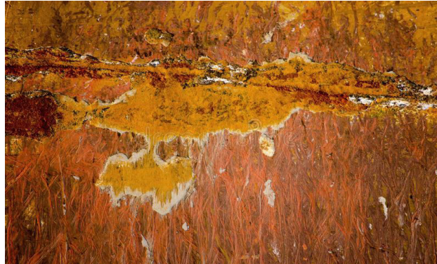
Fig.4. Intensive weld seam corrosion[8]
