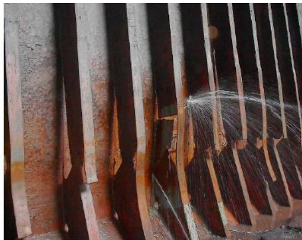
Fig.5. Intensive plating corrosion[8]
