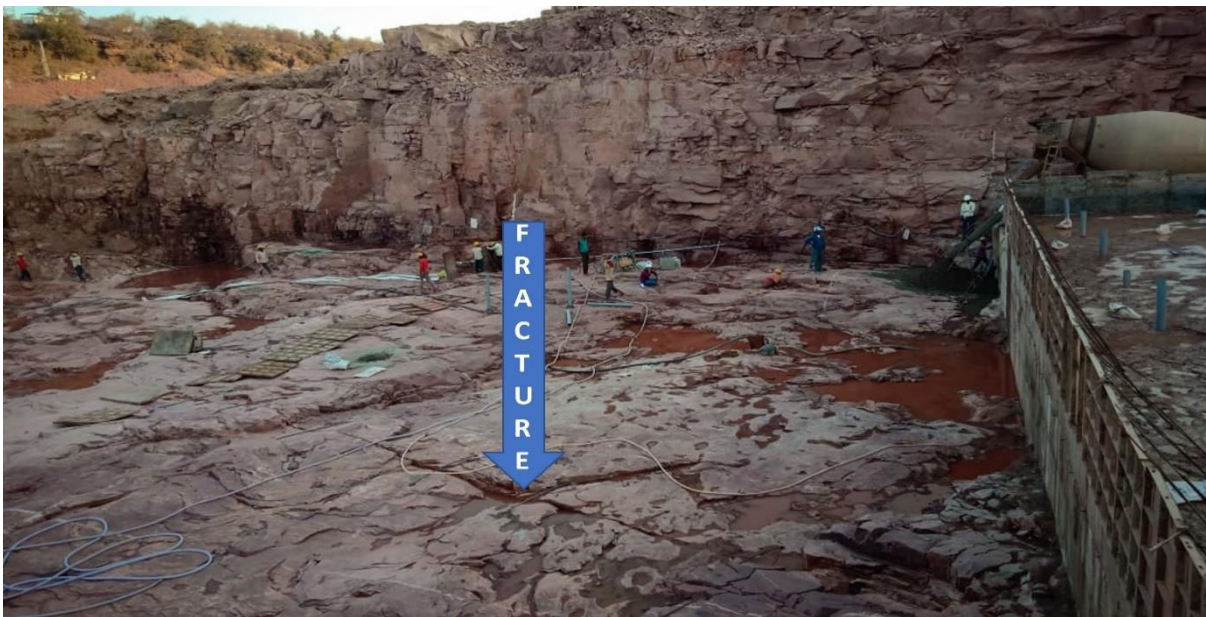
Figure 3: Fracture/ Shear Crack in Dam foundation
