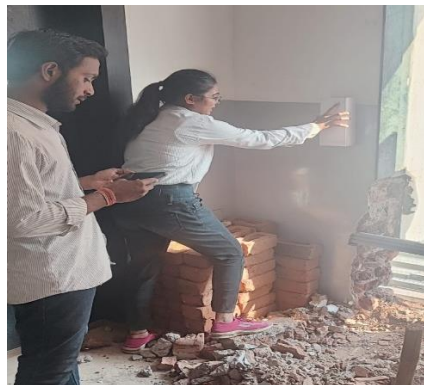
FIG. NO.11 DEMOLISHED STRUCTURE
