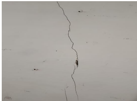
FIG.NO.9 LOAD BEARING WALL (DAMAGED STATE)
