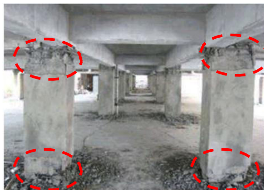
Figure 1.4 Plastic hinged formation at column ends of the ground storey columns in China Earthquake 2008
