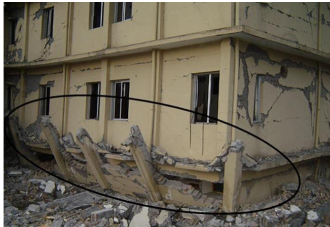
Figure 1.3 Shear failures of ground storey columns (Ref. World Housing Encyclopedia, EERI & AIEE)
