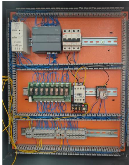
Fig. 3. PLC Panel board
