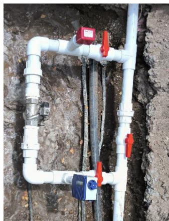
Fig. 6. Plumbing setup with sensors
