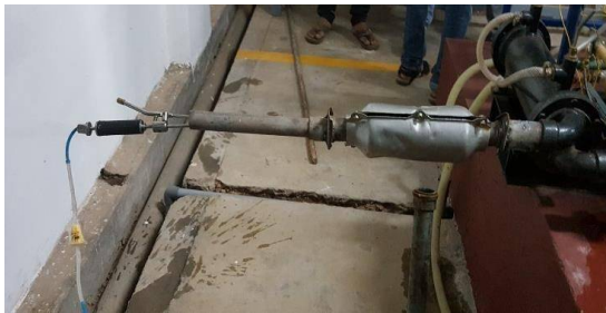
Fig. 2.7 : Gas analyser connection to engine
