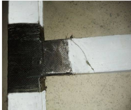
Fig. 8. Crack Pattern of BCJ CF-01
