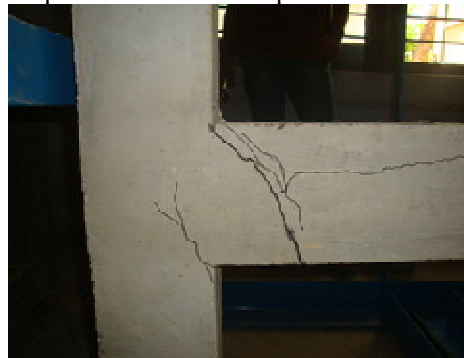
Fig. 7. Crack Pattern of BCJ
