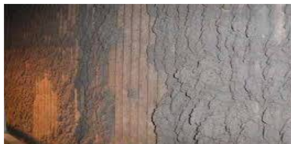
Fig. 2.4. Slag formed around boiler tubes
