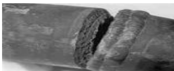
Fig. 2.7 Dissimilar metal weld failure
