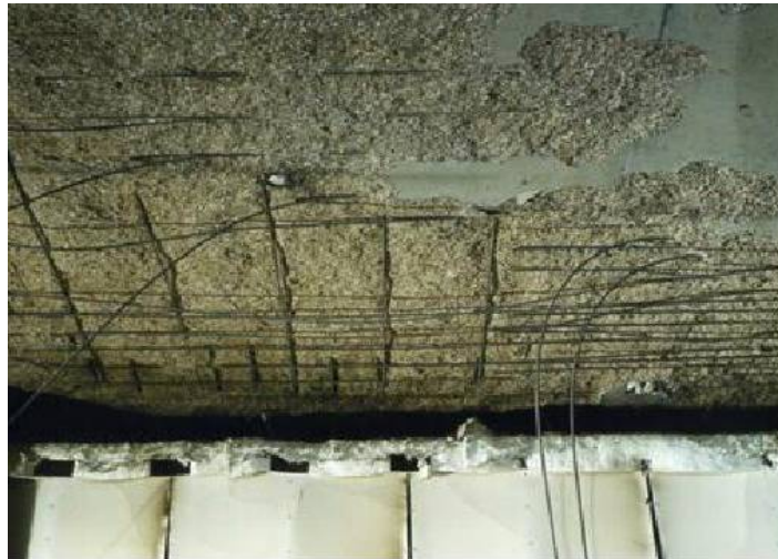
figure 1 (Showing spalling of Concrete)
