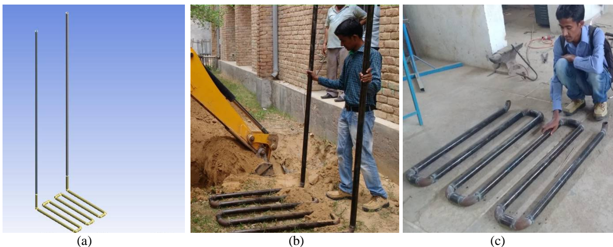
Fig. 1. Geometry of EATHE in Series Connection (a) ANSYS Geometry (b) Installation of Setup (c) EATHE in Series Connection
