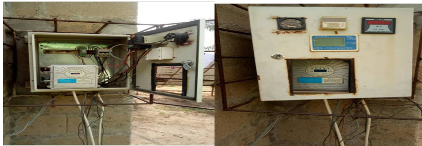
Plate 2: Instruments Control System Measuring Voltage, Current, Temperature and Discharge Rate.
