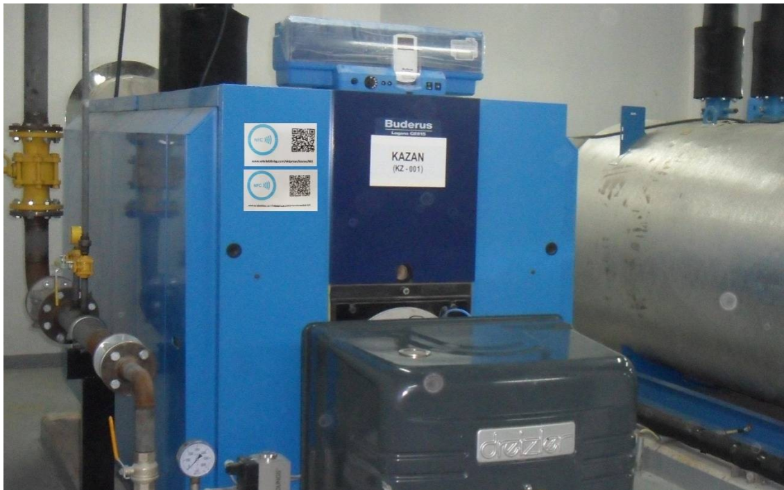
Figure 5. Picture of tags applied on the boiler.
