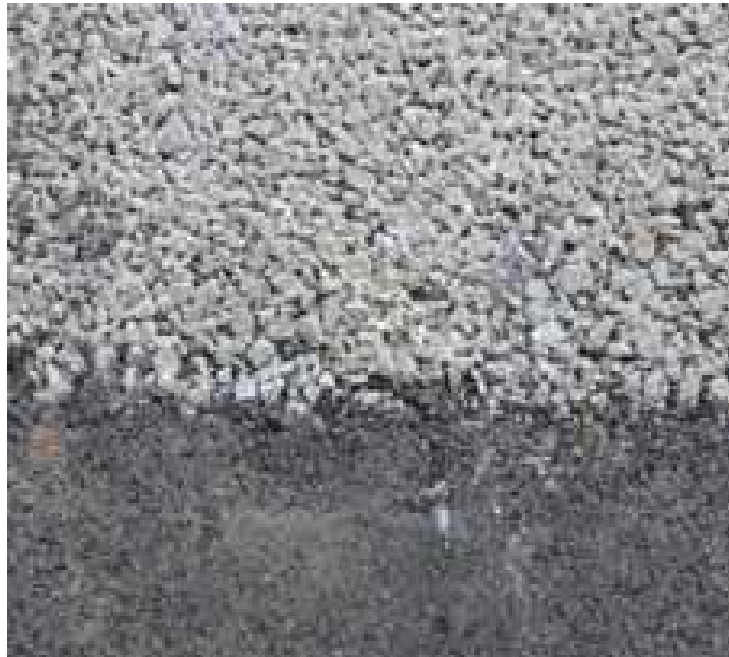
Figure 1. Permeable pavement (upper portion of figure) has large void spaces to allow water to infiltrate, unlike traditional asphalt (lower portion of figure).
