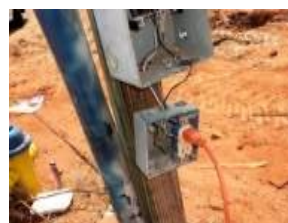
Exposed electrical parts
