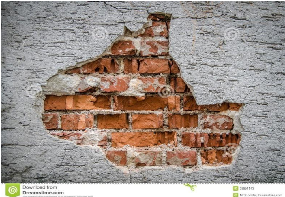
Figure 1.2 Plaster Damage (Non-Structural Problems)
