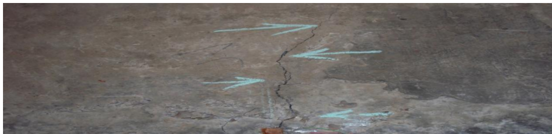
Fig.6 Crack Propagation in Beam
