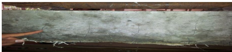
Fig.8: Failure of beam HSB-2
