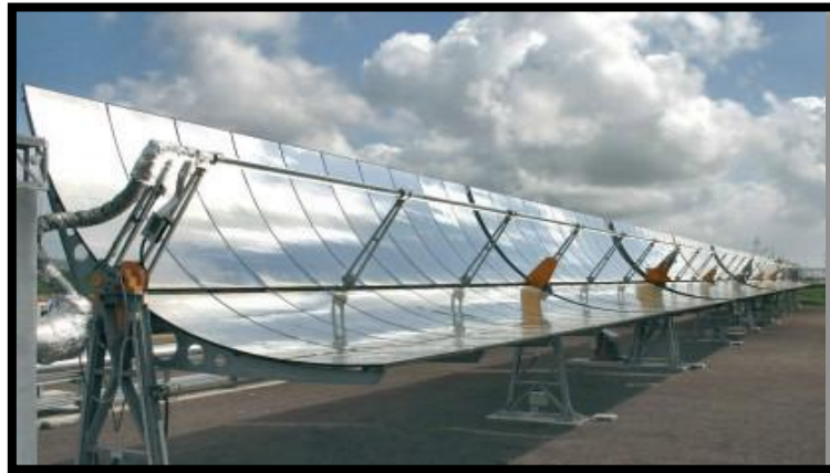
Figure-1: CSP Parabolic Trough Solar Collectors [2]
