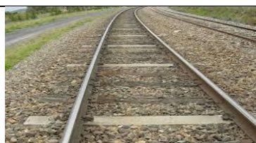
Fig 1.2 Prestressed geopolymer concrete railway sleepers installed as spot-replacement sleepers in the Melbourne to Sydney mainline, near Goulburn,NSW, Australia.(2005)
