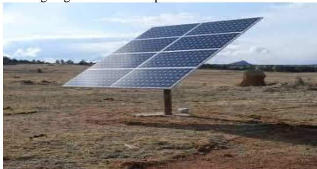
Fig.4 Photovoltaic System with Tracked Solar Panels
