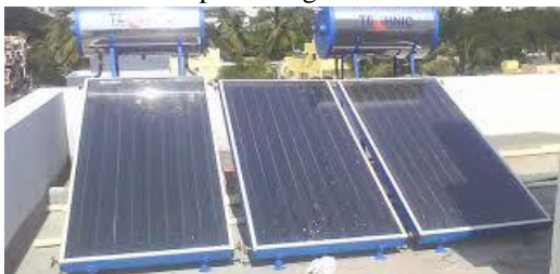
Figure 8: Passive solar hot water system on a residential roof top
