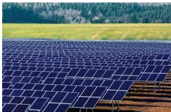
Figure 5:600 MW Solar Plant, Gujarat
