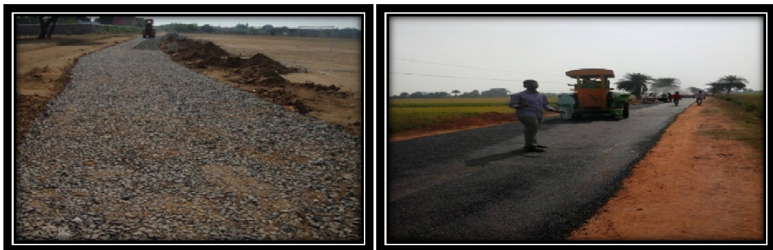
Fig 5. Laying of aggregates for W.B.M. roads and typical section for a bituminous, W.B.M. pavement. After placing the heavy aggregates, in the next process the small aggregates are placed and they are compacted by the road rollers. After attaining the good compaction, the bituminous is sprayed and leveled.
