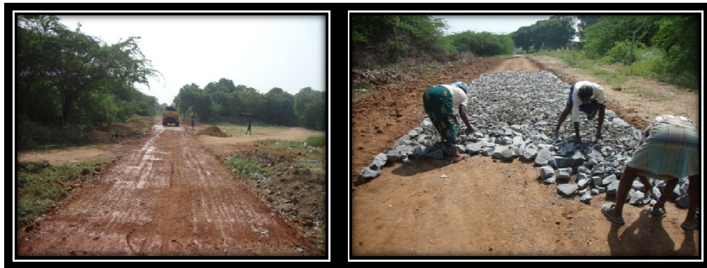
Fig.4. Typical section of a W.B.M. pavement is shown in the above figure and laying of aggregates for W.B.M. roads. The water is poured on the soil for a good compaction; usually the water is added by checking the optimum moisture content of the soil. The aggregates are placed in order, so that no bumps are formed later due to heavy compaction.
