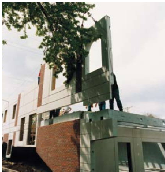
Figure 1: Panel-to-panel connections were designed to expedite construction of the University of Nebraska Duplex housing complex in Nebraska.
