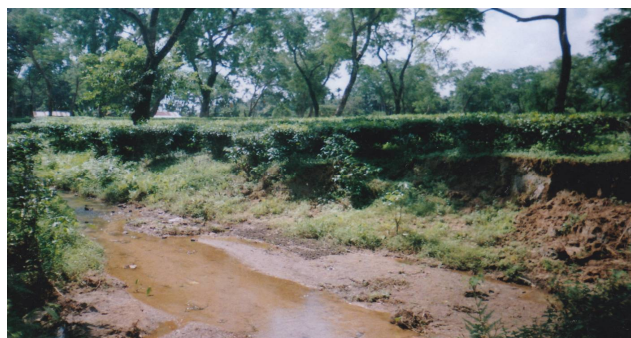
Fig. 1. A badly eroded drain.
