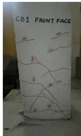
Fig. 7(a). Flexural cracks in CB1
