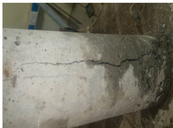
Figure 6. Failure of column
