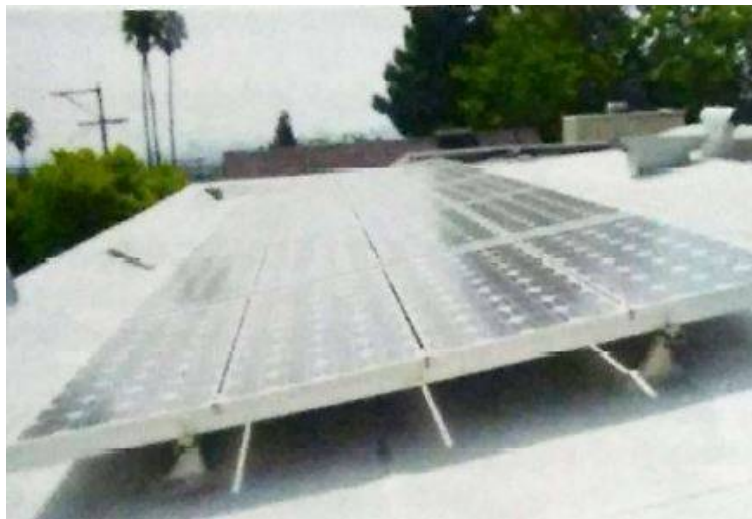
Fig 3: Solar panel set up
