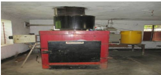
Figure 4.13: DMCH Incinerator Machine
