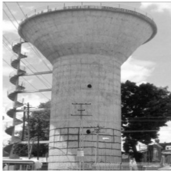
Fig. 2 Flexure cracks in staging
