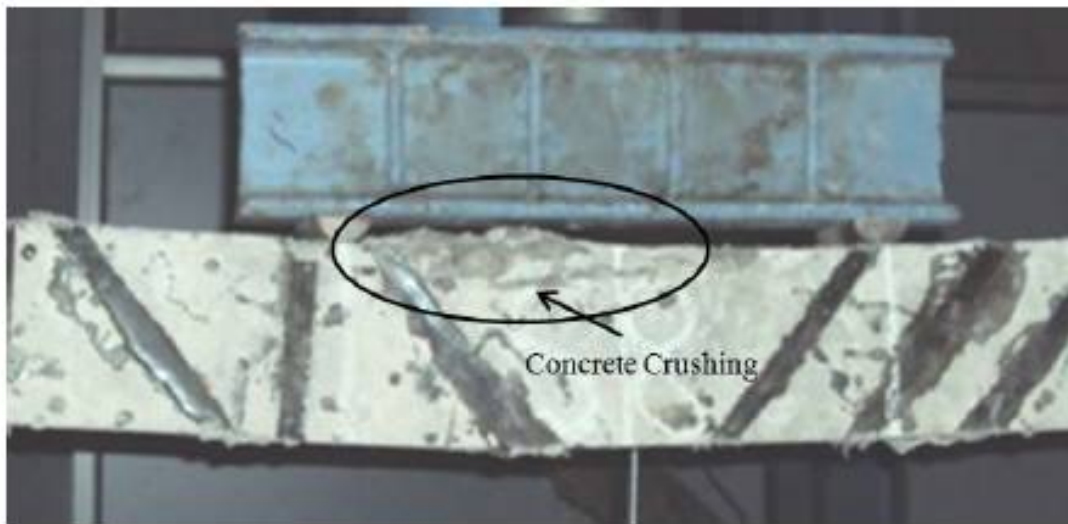
Fig. 3 Failure pattern of beam strengthened in shear using mixed pattern. Source: S. B. Singh et al (2014) [6]
