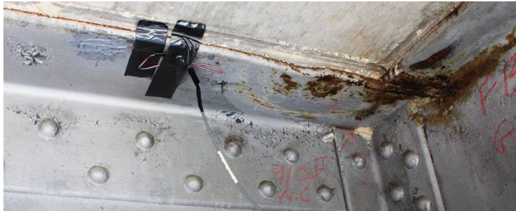
Strain gage located on the top flange of the longitudinal girder of Bridge approximately 2 ft away from the connection of the floor beam.
